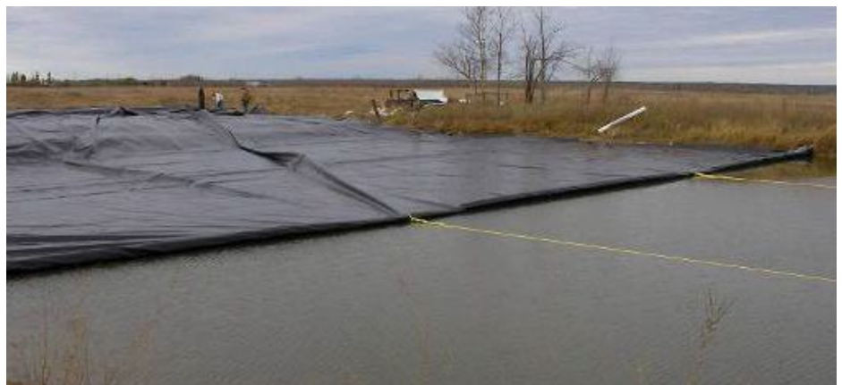
Figure 8. Floating Cover being pulled into place with rope and reinforced leading edge.
