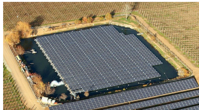
Figure 8. Open water floating solar (CN) (Image: PV Magazine USA, 2020)
