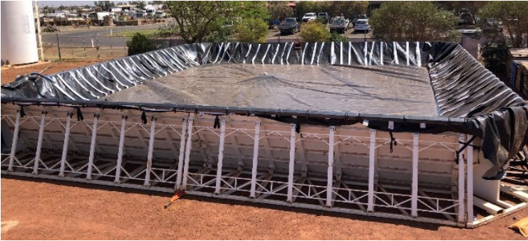
Figure 5. 0.75mm proprietary polyolefin rain cover on a coal seam gas frac storage to eliminate rainfall intermingling with stored fracking liquid. NT, Australia. (Image: MPC, 2018)
