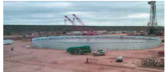
Figure 20. Enviro Liner® 6030 Frac Tank Liner, West Texas.
