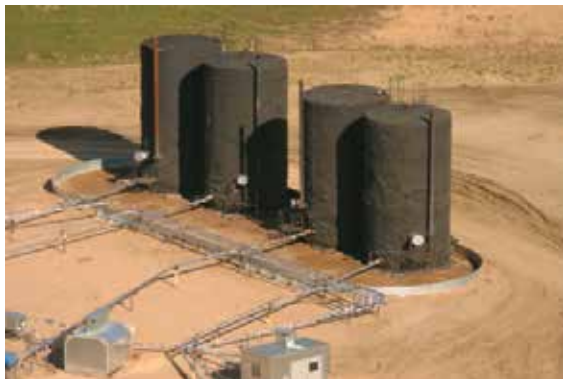
Figure 22. Secondary containment system in Alberta, Canada
