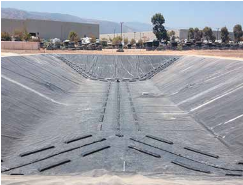
Figure 25. Reclaimed water storage reservoir floating cover fabricated with Enviro Liner® 6060, Corona California
