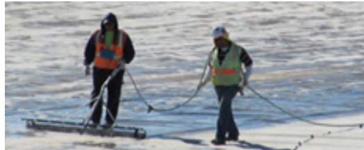
Figure 5. Water Puddle Testing
