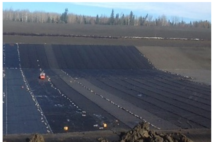
Figure 3. Geovolt® placement on the site
