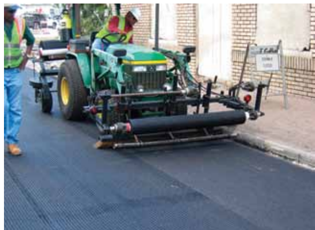
A GlasGrid full width installation using a high speed, 5 ft wide installation device.
