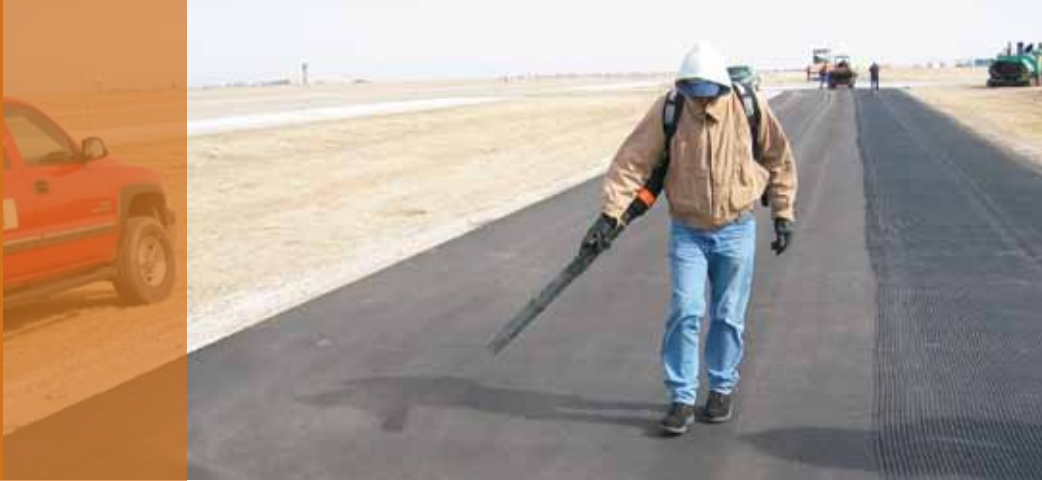
Surface preparation includes blowing off any dust before installing the self-adhesive GlasGrid System.
