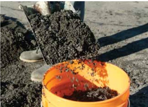
IMAGE A: Milled asphalt containing GlasGrid product can be easily recycled for use on other projects.
