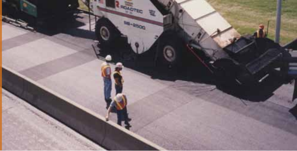
GlasGrid detail repair installation where an asphalt transfer device is used as part of the paving train.
