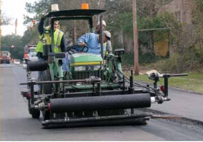
Five foot wide GlasGrid rolls allow for rapid installation due to ease of handling and less manpower.
